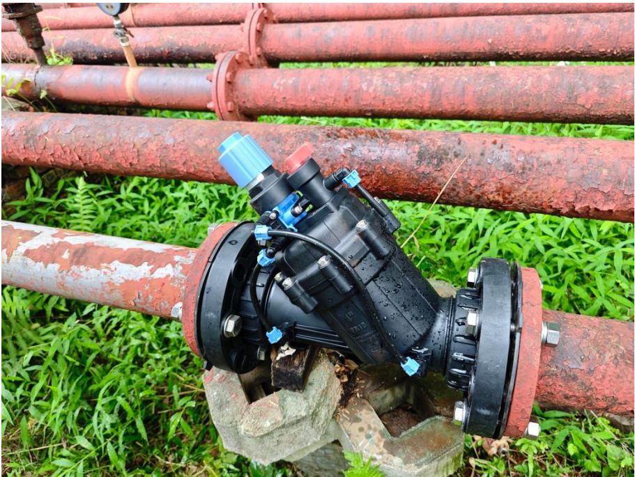
Runjing Pressure Relief Valve Applied to a Golf Course in Wenzhou, Zhejiang
